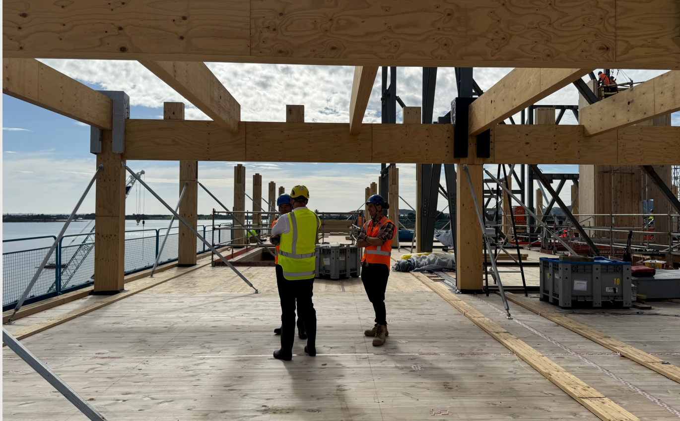
A view of the mass timber frame elements during construction at 90 Devonport Road, Tauranga
